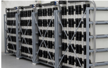
Energy Storage System
