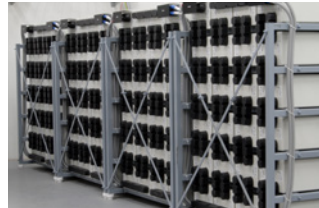
Energy Storage System
